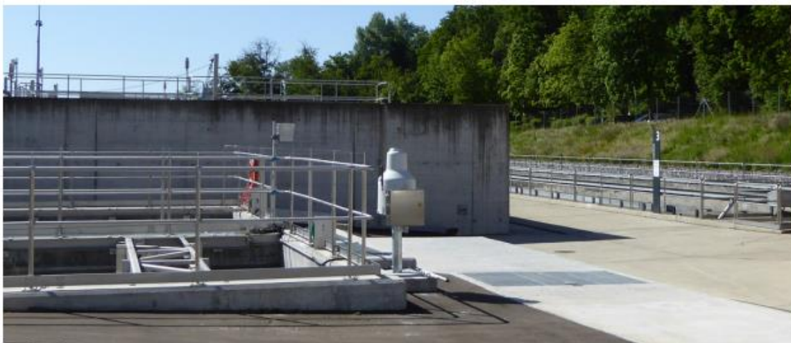
Foto der Station Uster (UST)
